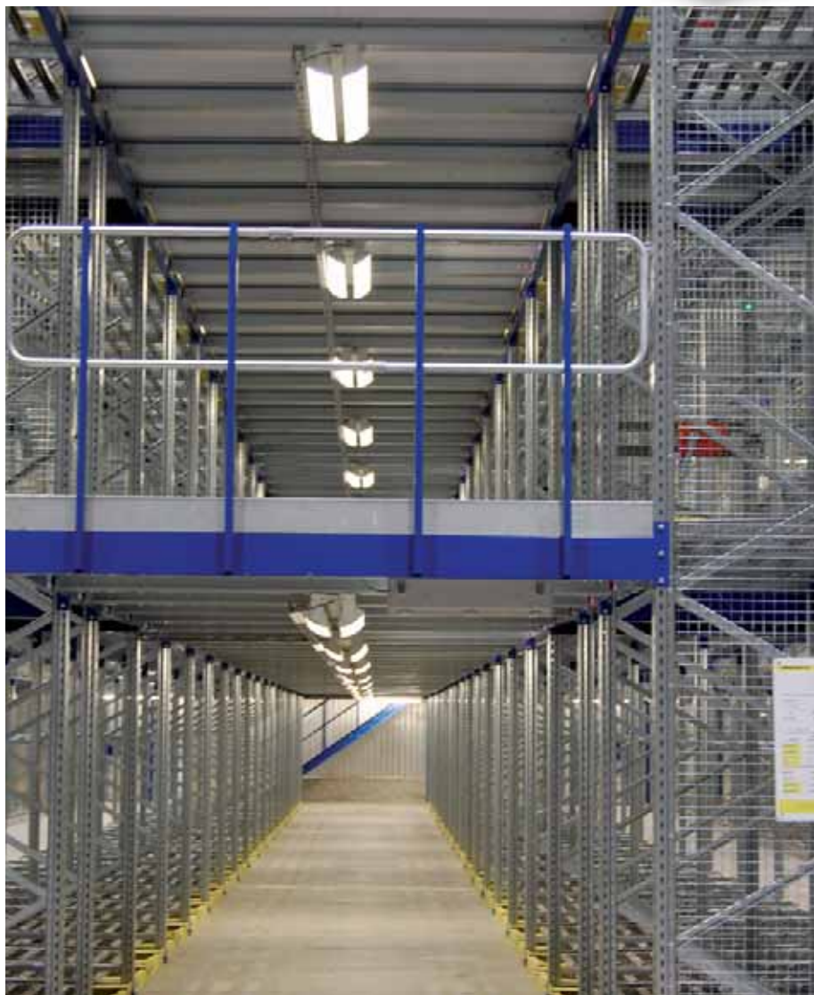
TURKU LED luminaire, single lamp, with reflector tube, PMMA clear, 80 lm/W, 5400 K
